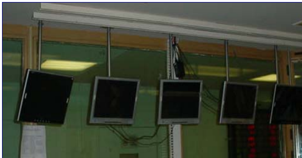
Monitors in the Command Center allow a view of activity throughout the CDF.
